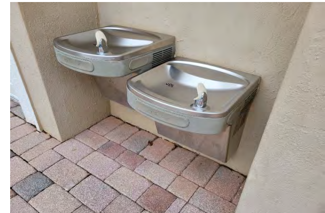
Patio Furniture & Drinking Fountain
