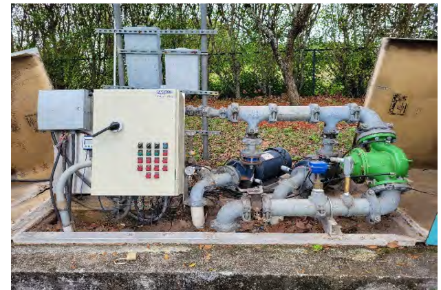
North Irrigation Pump Station
