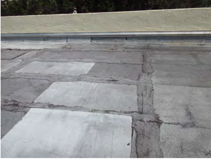
VIEW OF FAILING ROOF MEMBRANE
