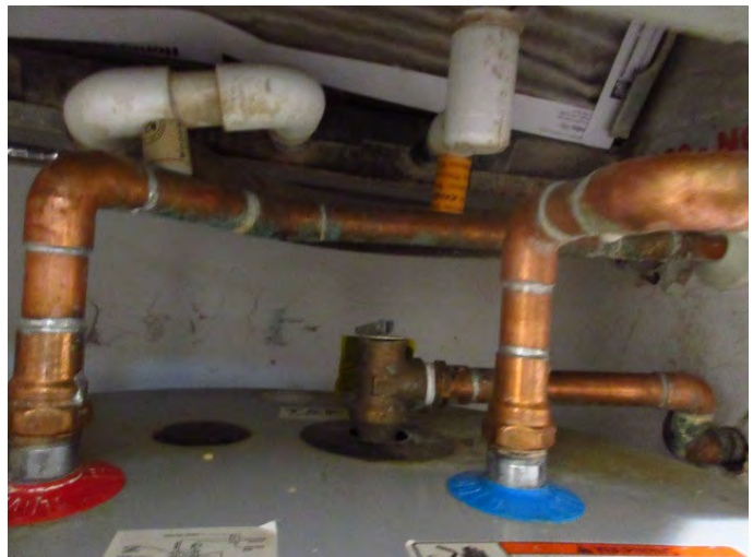
VIEW OF DOMESTIC WATER COPPER PIPING
