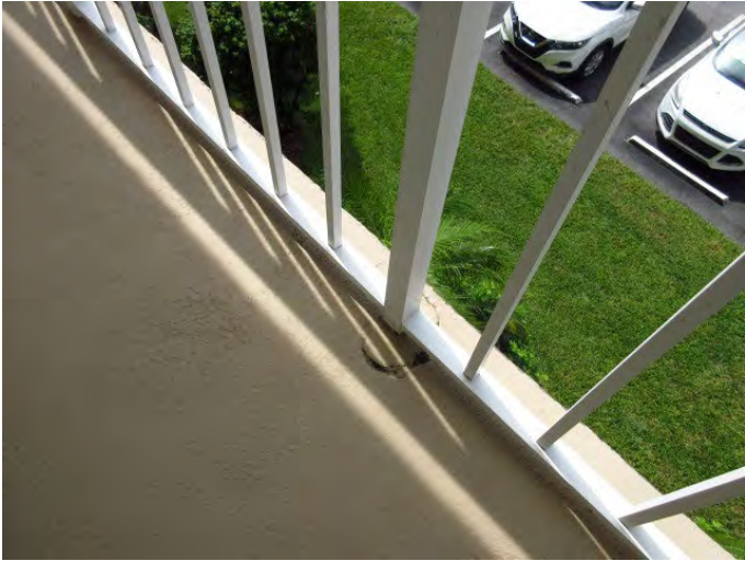
DAMAGED UPPER-LEVEL WALKWAY SLAB AT RAILING
