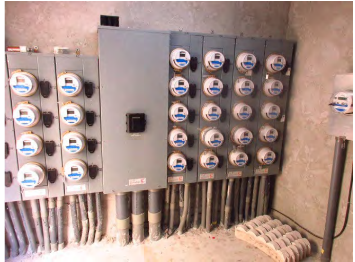
VIEW OF ELECTRICAL EQUIPMENT
