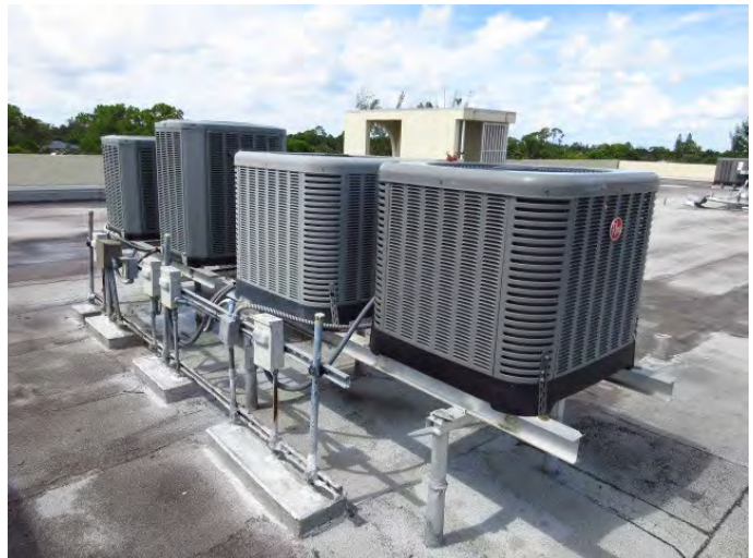
VIEW OF HVAC EQUIPMENT
