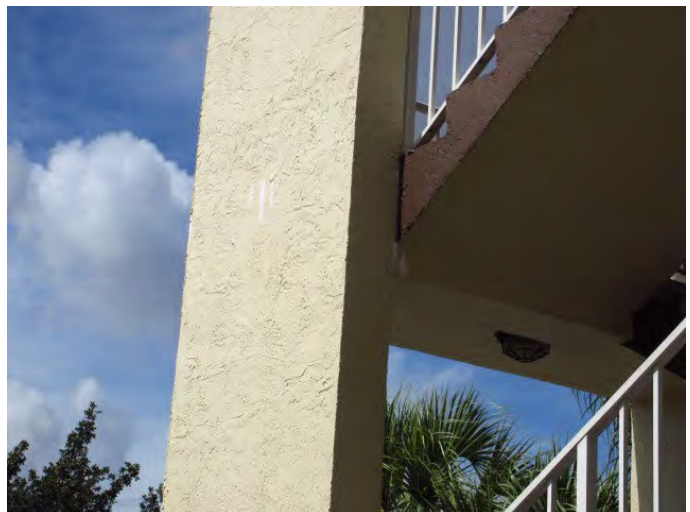
MINOR EFFLORESCENCE ON FAÇADE
