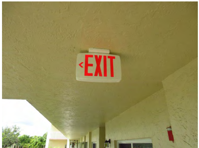
VIEW OF LIFE / SAFETY EQUIPMENT
