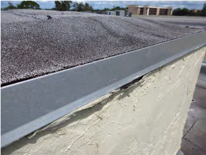
VIEW OF DAMAGED EXTERIOR WALL
