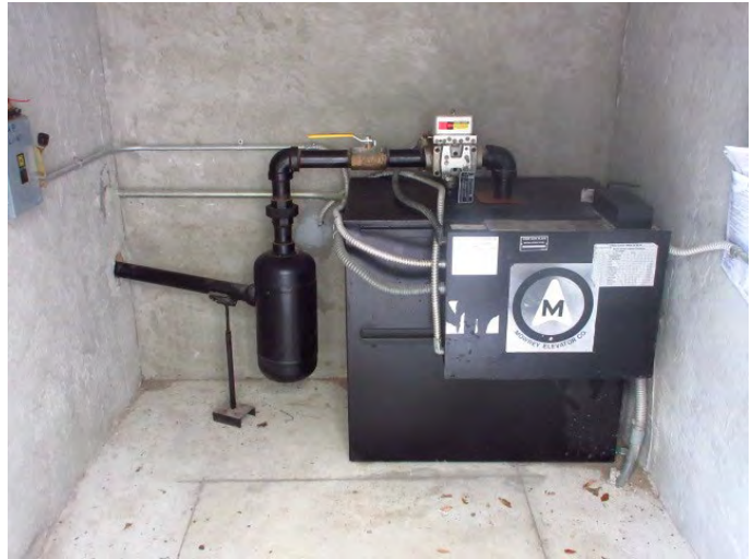
VIEW OF ELEVATOR EQUIPMENT
