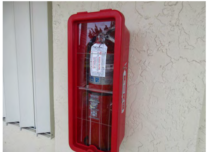
VIEW OF FIRE EXTINGUISHER
