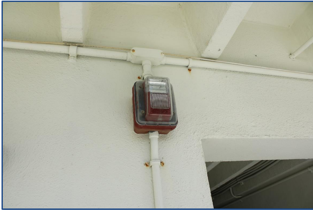
Photograph No. 13: Common area fire alarm.
