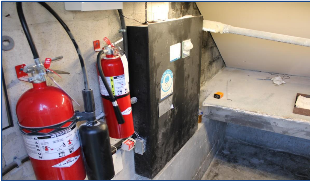
Photograph No. 15: Fire extinguishers.
