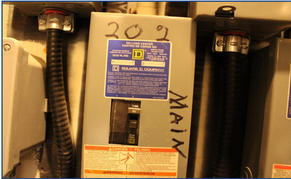
Photograph No. 19: Main switch for individual units.
