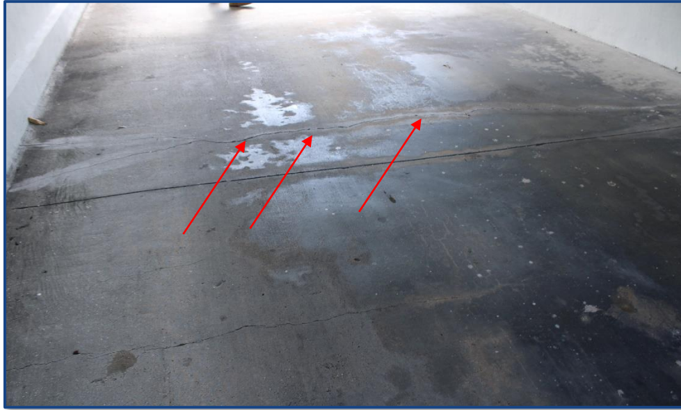
Photograph No. 21: Building driveway crack.
