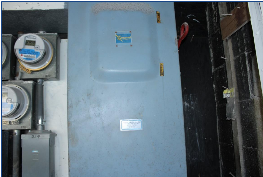
Photograph No. 20: Main electrical panel switch.
