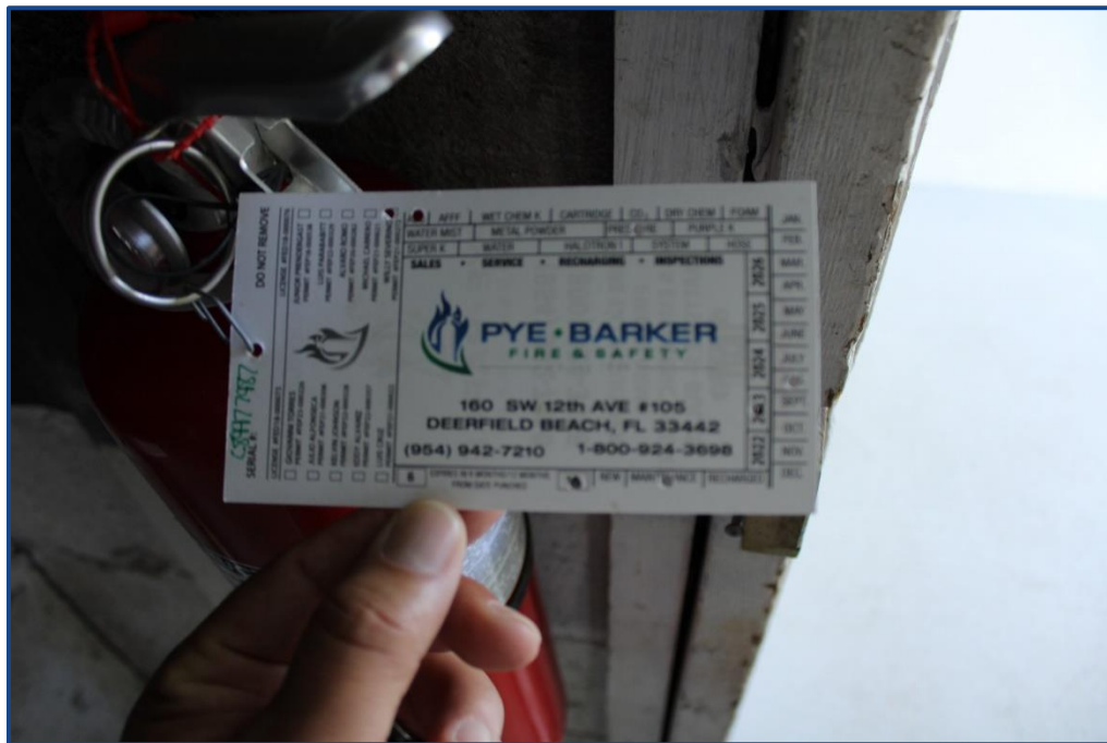
Photograph No. 16: Fire extinguisher inspection card.
