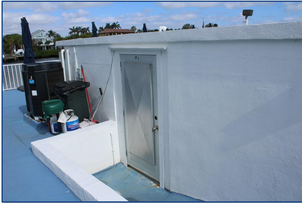
Photograph No. 7: Pool equipment room.
