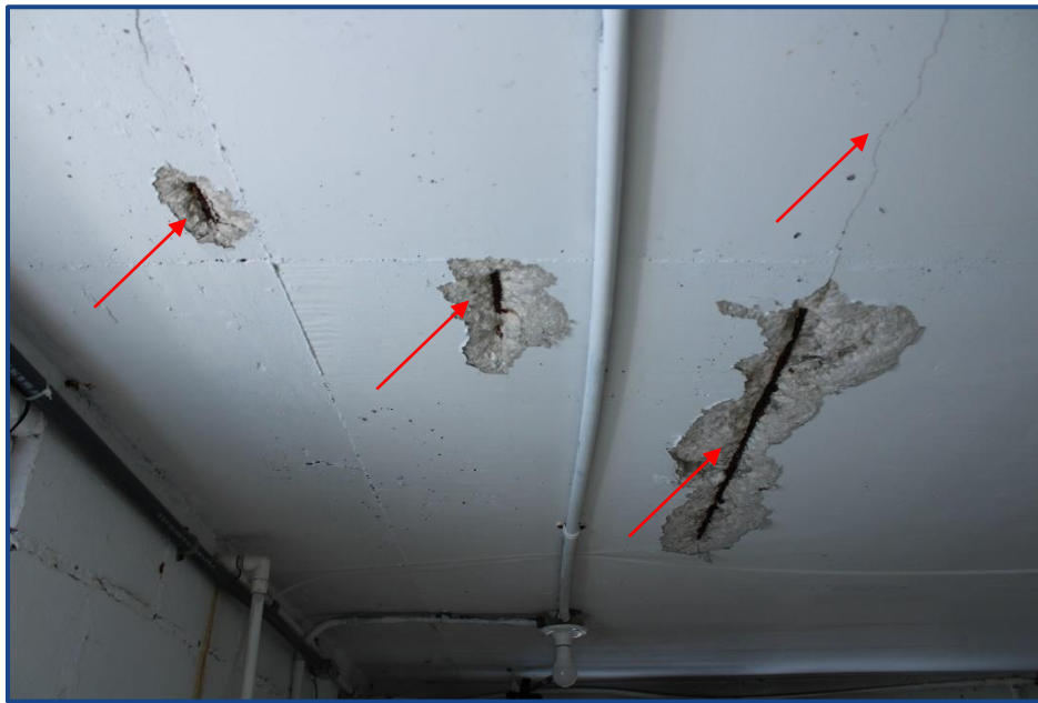
Photograph No. 10: Concrete spalls and cracks at the ceiling of the pool equipment room.
