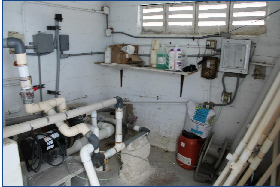
Photograph No. 9: Pool equipment.
