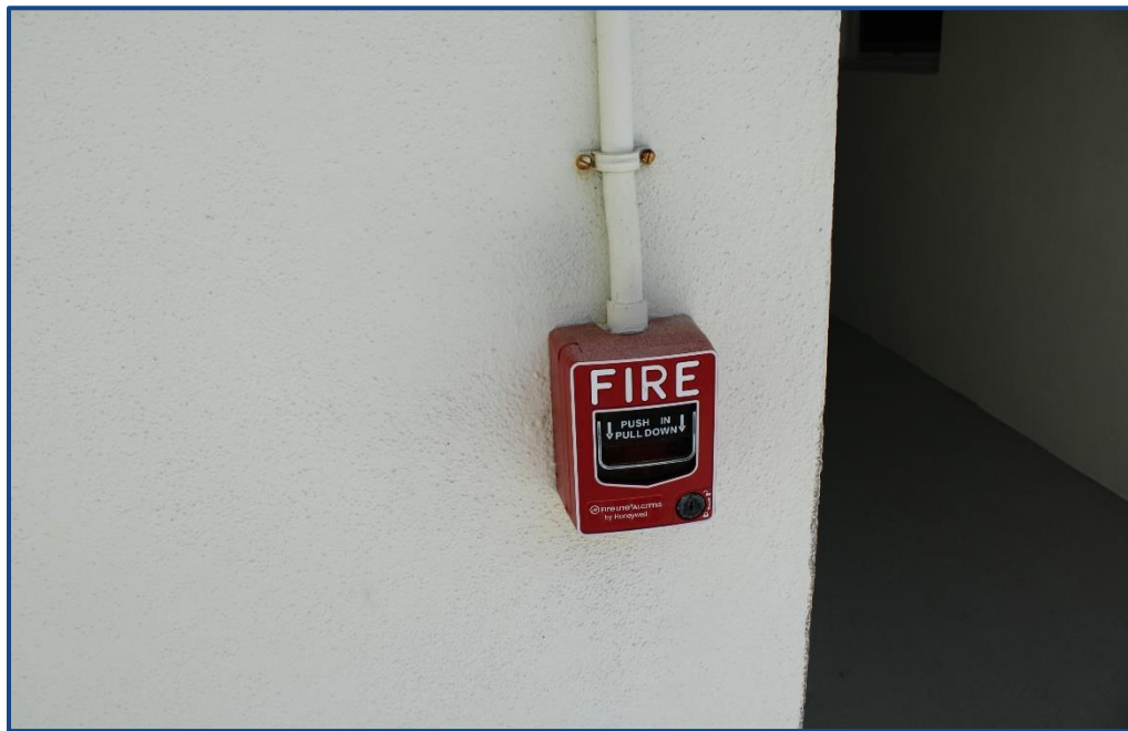
Photograph No. 14: Common area fire alarm switch.
