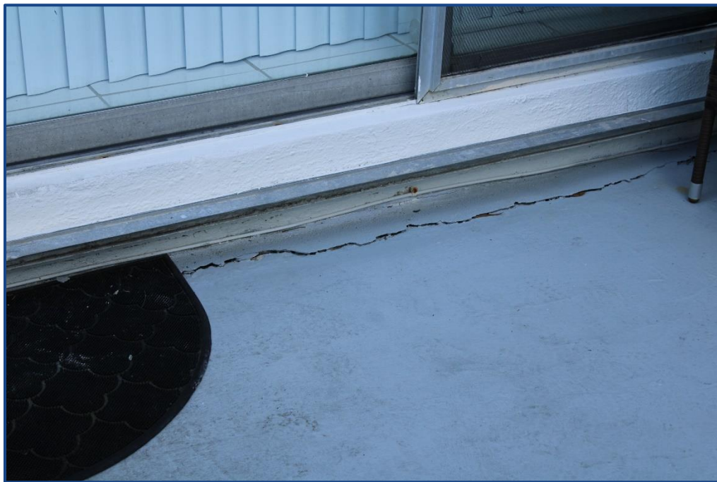
Photograph No. 24: Concrete crack at exterior patios, typical.
