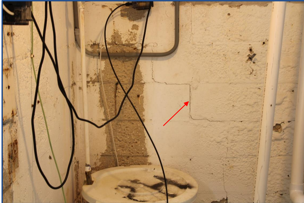
Photograph No. 8: Crack in the interior wall of the pool equipment room.
