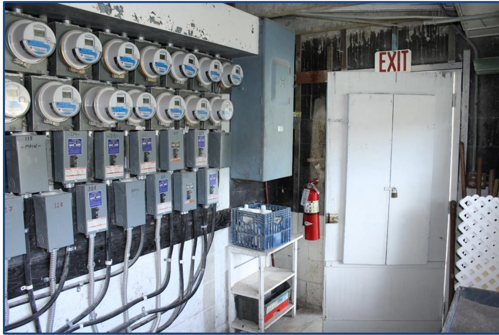
Photograph No. 17: Electrical meter room.
