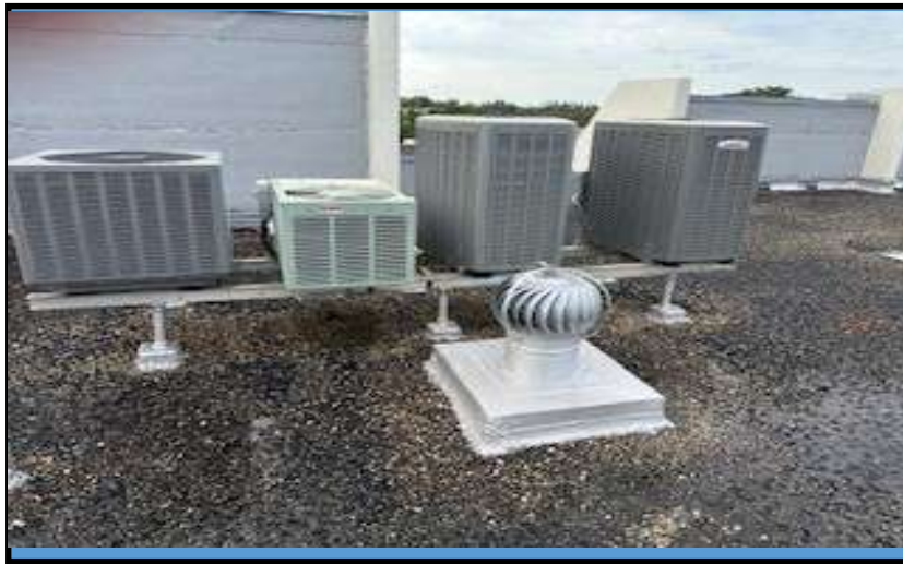
TYPICAL PLATFORM ELEVATED AIR CONDITIONING UNITS AND ROOF VENT
