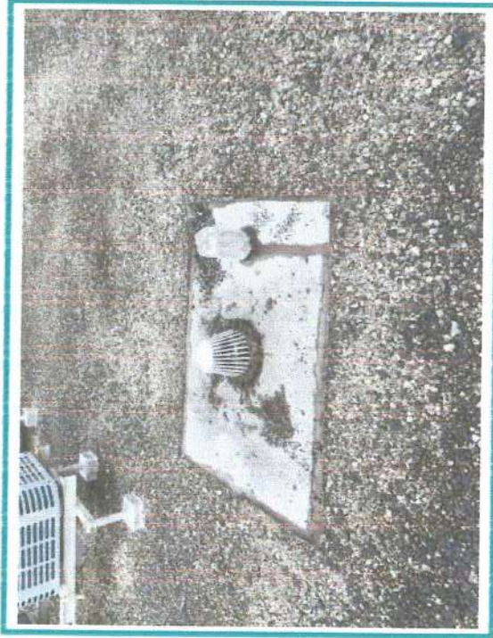
9. View of typical interior drain detail, boarder needs coating
