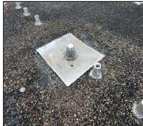
TYPICAL ROOF DRAIN
