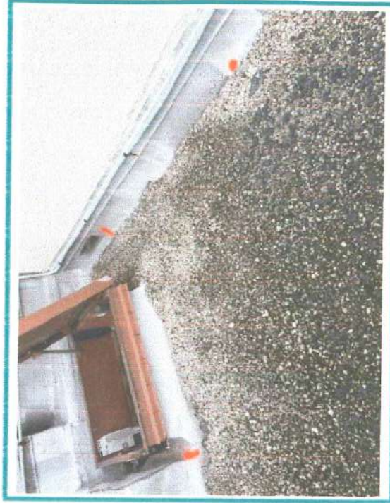
12. Small isolated area of subsurface water adjacent to hatch
