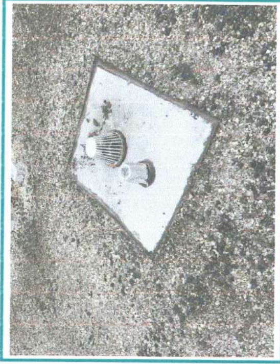
14 View of typical interior drain detail, boarder needs coating
