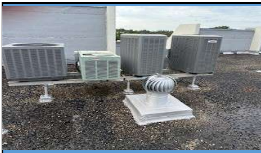
TYPICAL PLATFORM ELEVATED AIR CONDITIONING UNITS AND ROOF VENT
