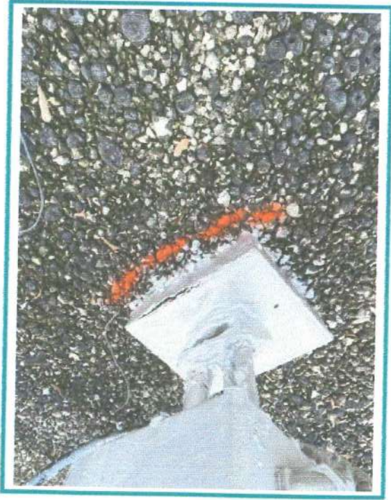
13 Penetration pan slightly separated from fill, repair
