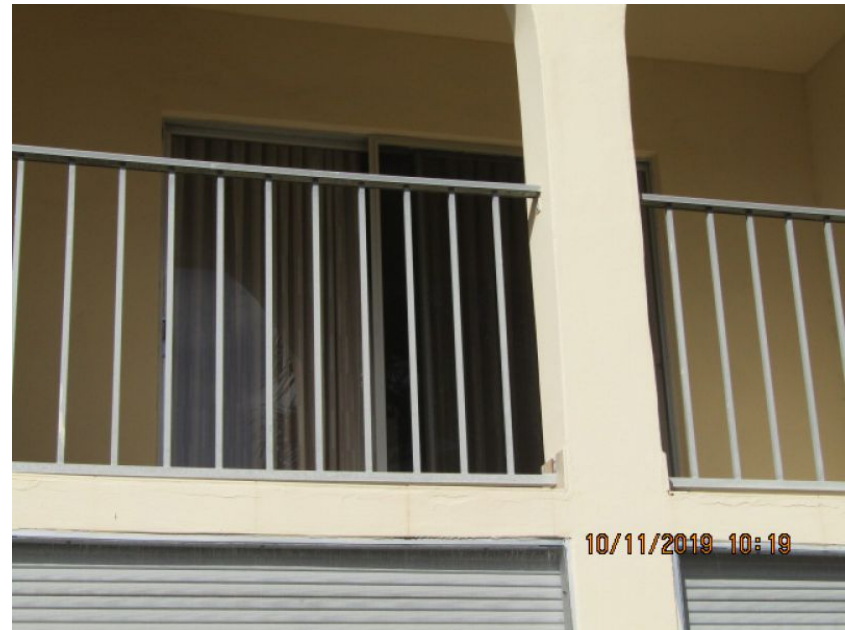
Unprotected Glazed Entry Door
