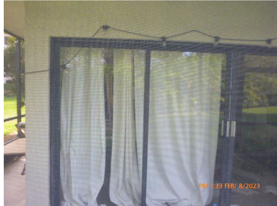
Unprotected Glazed Door
